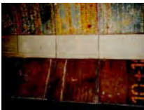
Clinker breaker housing
