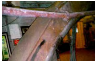
Raw mill transport pipe
